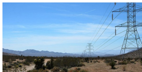
Transmission line leading to the Lugo substation | Edison International
